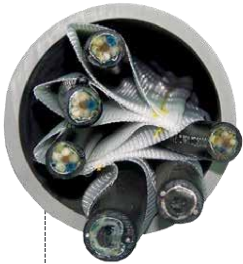
2" 3-Cell packs, 6 cables in 3" conduit
