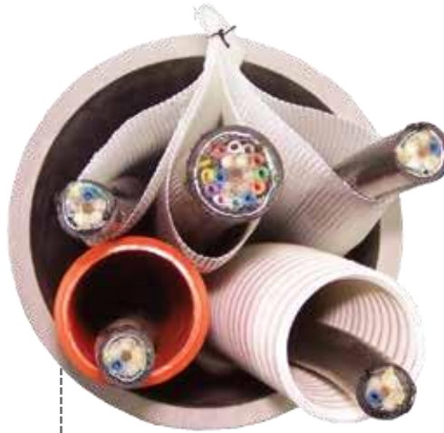
3" 3-Cell pack overriding existing cable plant in 4" conduit
