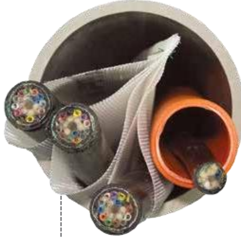
4" 3-Cell packs overriding existing cable plant
